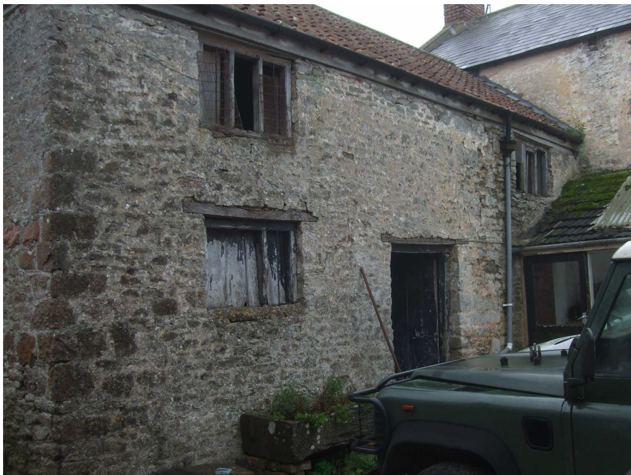
Fig 12: West aspect of north-east range with surviving windows of cider house, November 2012
