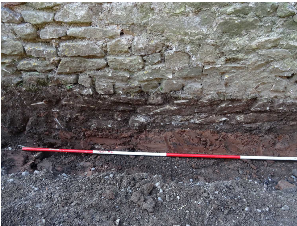
Fig 7: Trench alongside north-east range (broken ceramic pipes removed) showing shallow foundations (approx. 20-30cm) by soil mark on the walls: 12 April 2018
