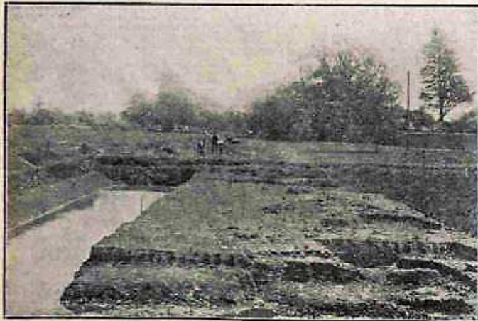
Diverting the course of the River Yeo by digging a new bed. The line of trees and wall show the present course of the river.
