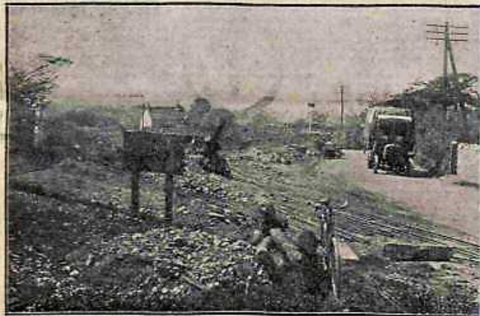
Cutting a new road at the top of Rhodyate looking towards Congresbury.
