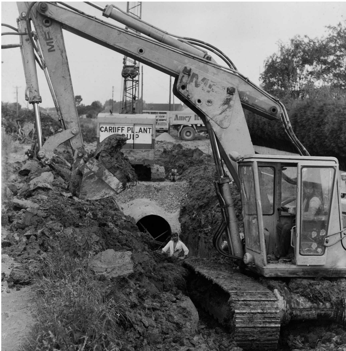
Culverting the Middle Yeo, Clevedon Town, 1960s (and risking instant dismissal under modern Health and Safety rules!) Photograph by Derek Lilly
